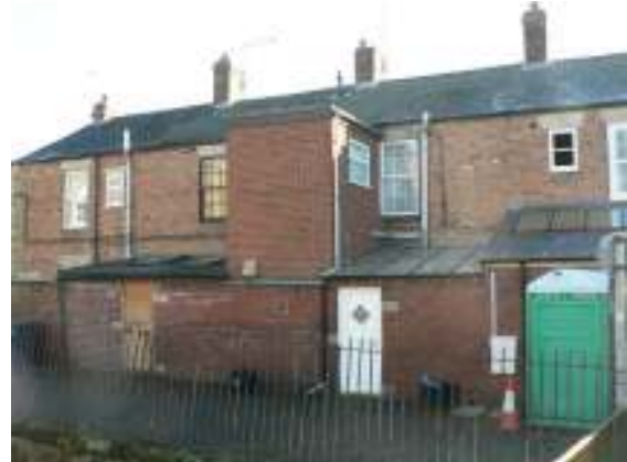
Inappropriate extension detracting from worker's cottage.
