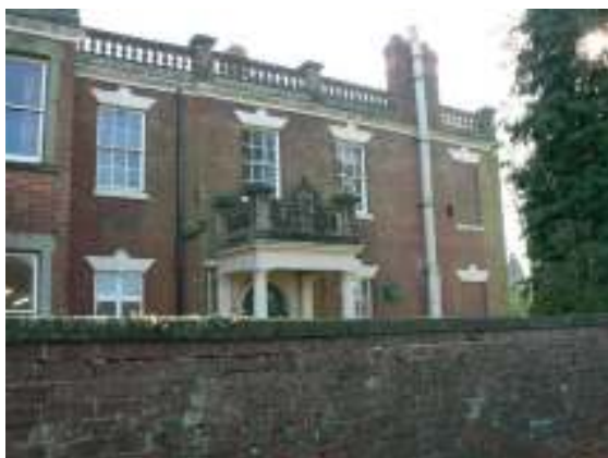
Attractive original sash windows significantly enhance the aesthetic appeal of the conservation area
