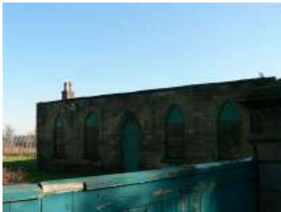
Boarded up structure in need of renovation
