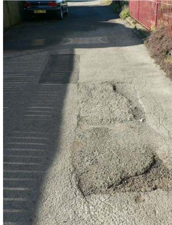
Poor paving needs to be addressed
